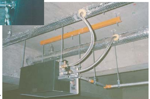
Ceiling Mounted FCU >
